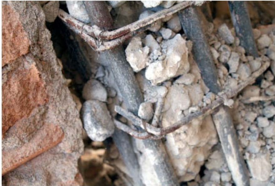
Figure 4: Failure according to stirrups with insufficient anchorage after earthquake action [8]
