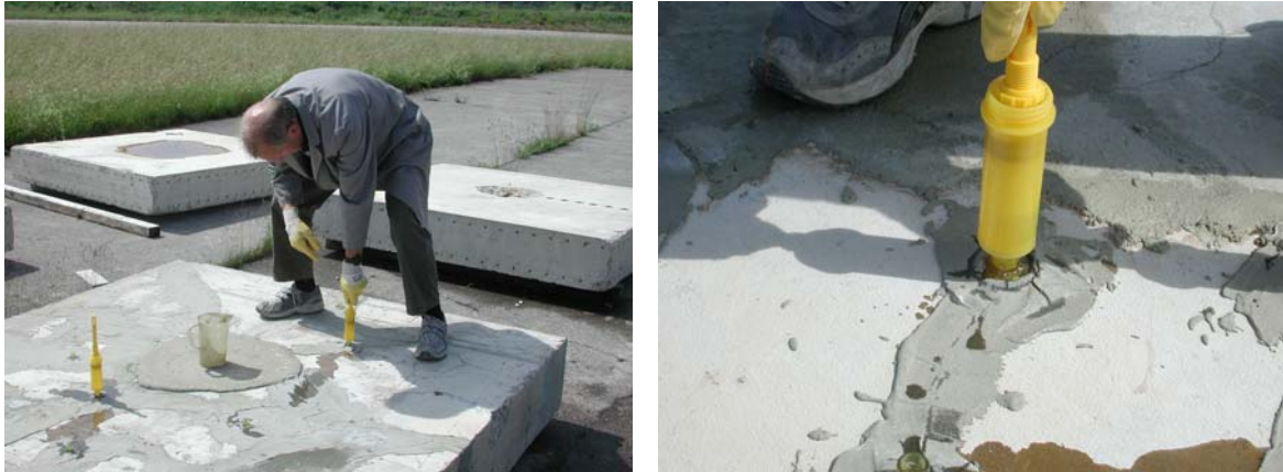
Figure 8: Use of epoxy grouting with low pressure injector for slabs loaded with contact detonation
